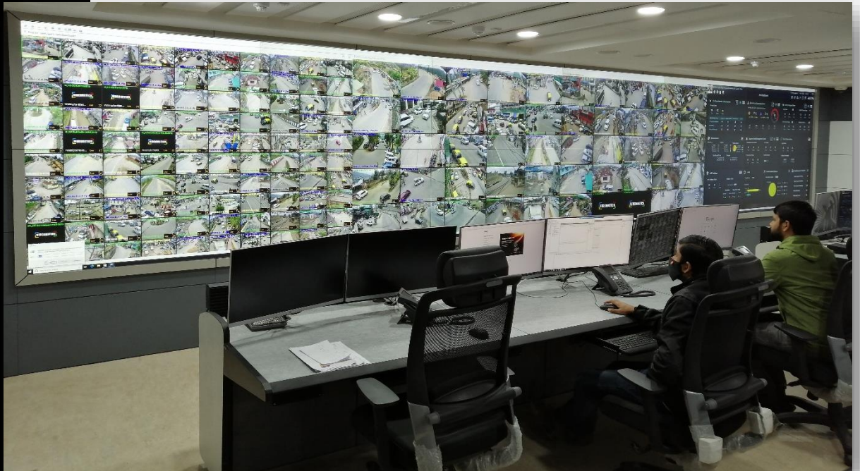
Smart City Integrated Command & Control Center
