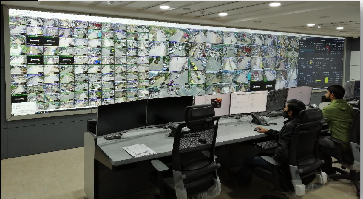
Smart City Integrated Command & Control Center
